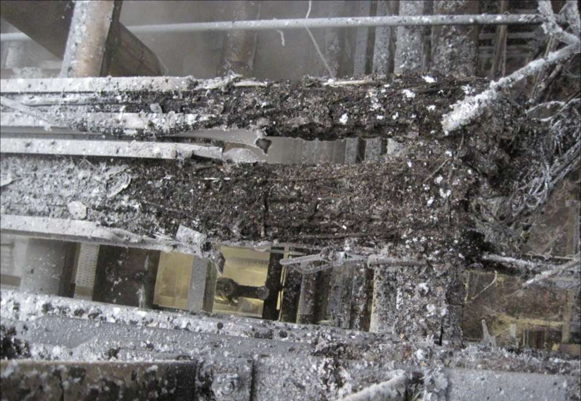
Example of tray / cable damage
