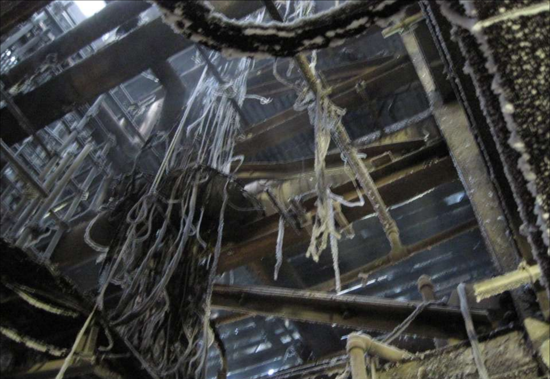
Example of tray / cable damage
