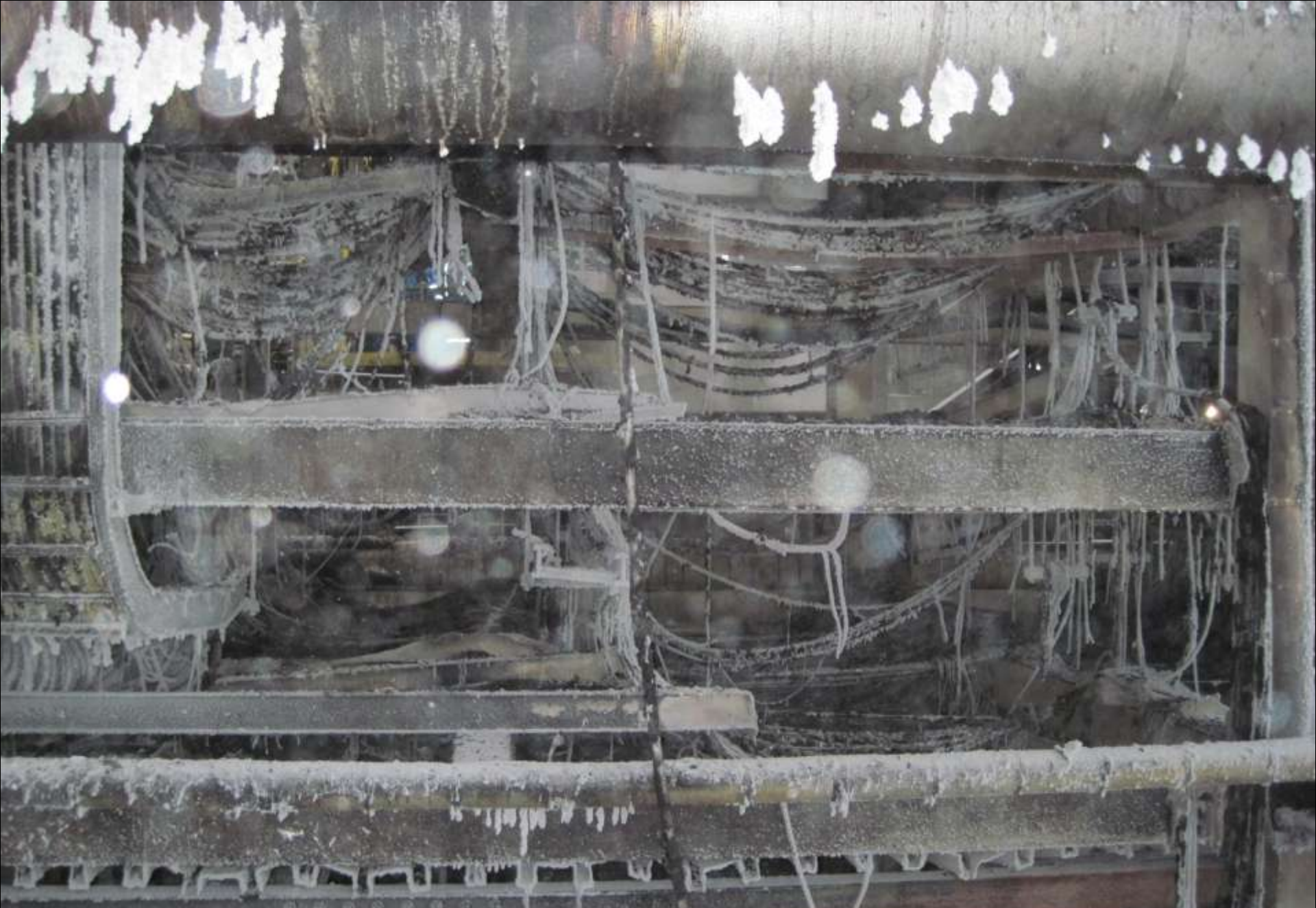
Example of tray / cable damage
